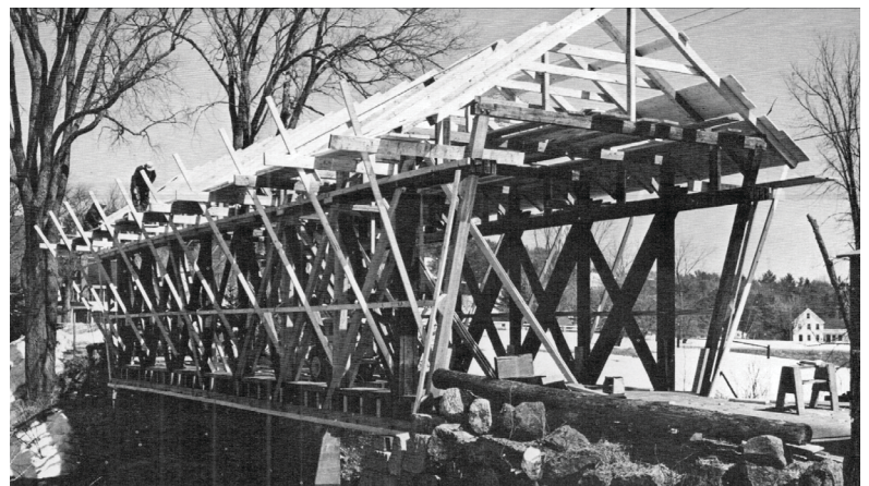
The 1968-69 repairs were extensive and included a new roof system and the replacement of many of the structural truss members.
