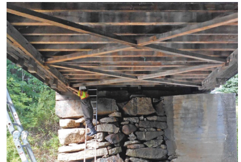
Under bridge inspection, 2017, shows a good view of the structure below deck.
