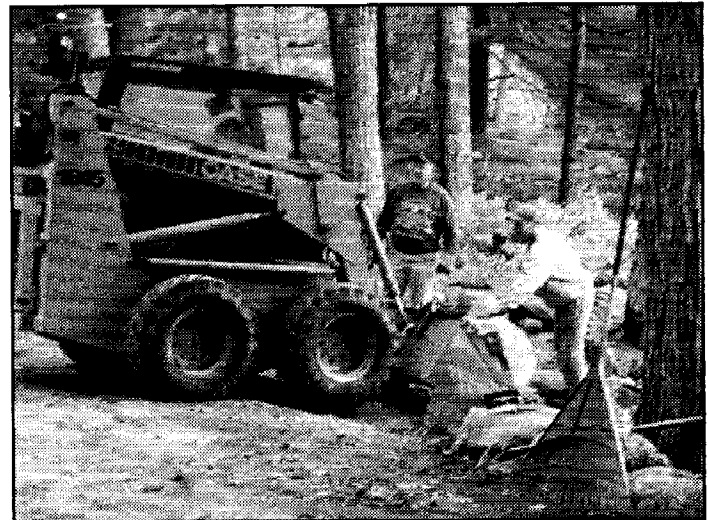
Jim Allen at the wheel, Wacky Lucas supervising and Jim Raymond doing the work
